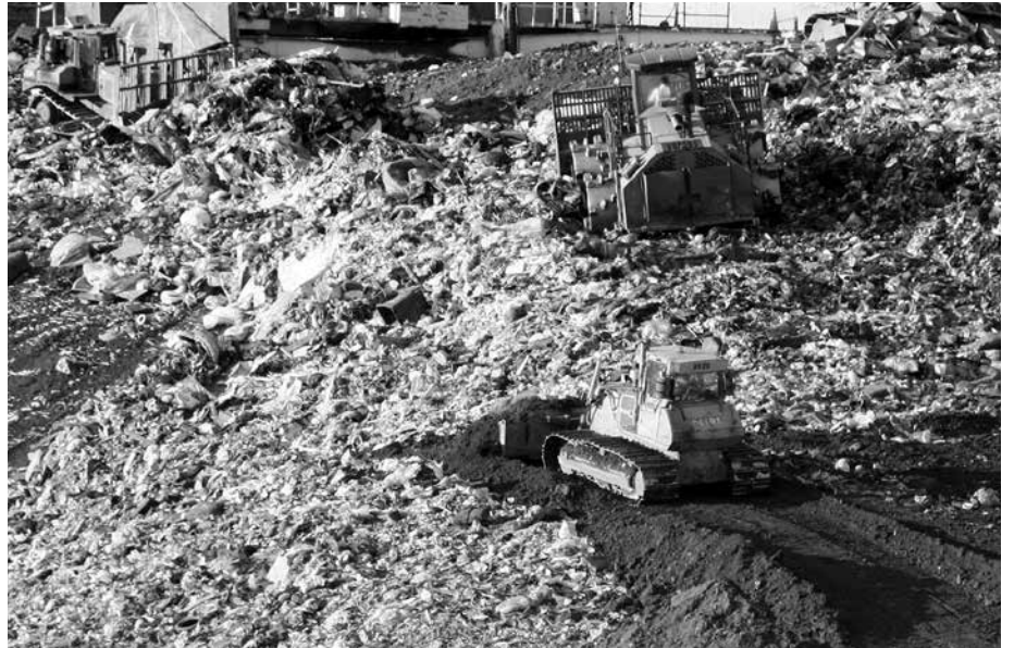
An open cell at Casella Waste Systems, Inc.'s NEWSVT Landfill in Coventry, Vermont. Because WEC produces electricity from the trash that's sent there, the content of the waste stream is a matter of importance to the Co-op.
