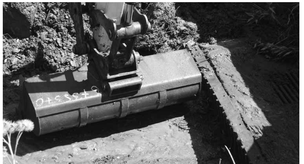
The heavy rains of July 19, which caused flooding in Plainfield and Barre, produced mud blockage of a drainage system behind WEC's office building. The Bobcat was able to maneuver into place and clear it out, then clean up the debris in WEC's parking lot.
