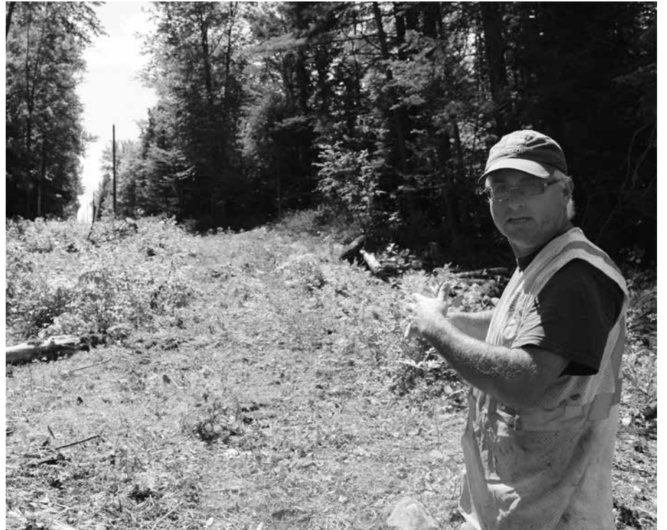
Mike Myers reveals a newly cleared right of way in a forested area of Topsham. This summer a storm took down two 1940s-era poles, and right of way crews and line crews worked to cut back dense growth and replace the poles and lines.
