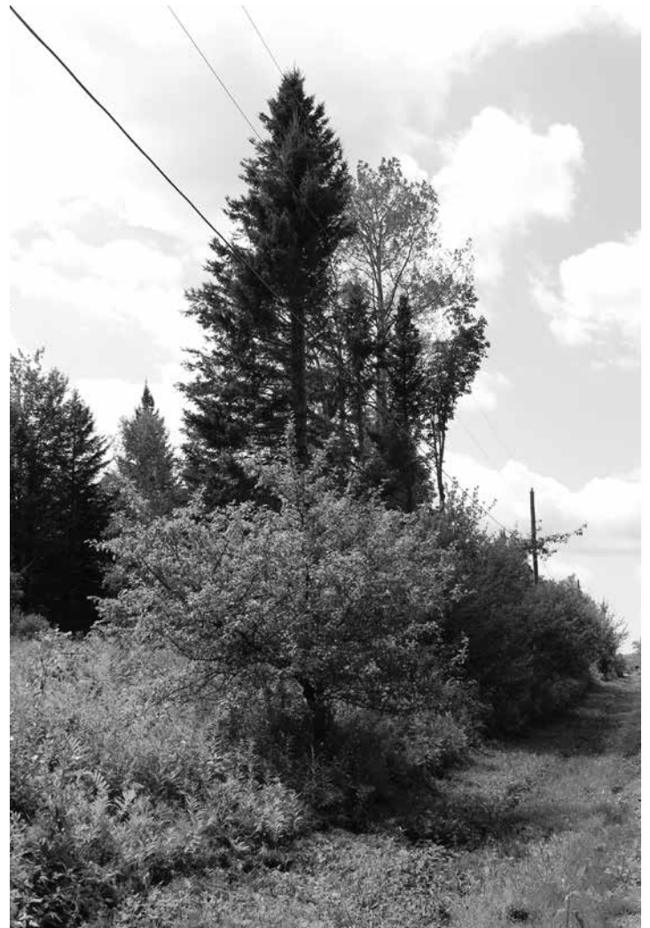
Right of way crews flat-cut under the line but took care to leave this homeowner’s apple tree standing.
