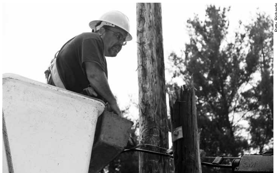
Larry Gilbert, First Class Lineworker, works to set a new pole next to one broken by the windstorm. WEC replaced 19 broken poles in all.
