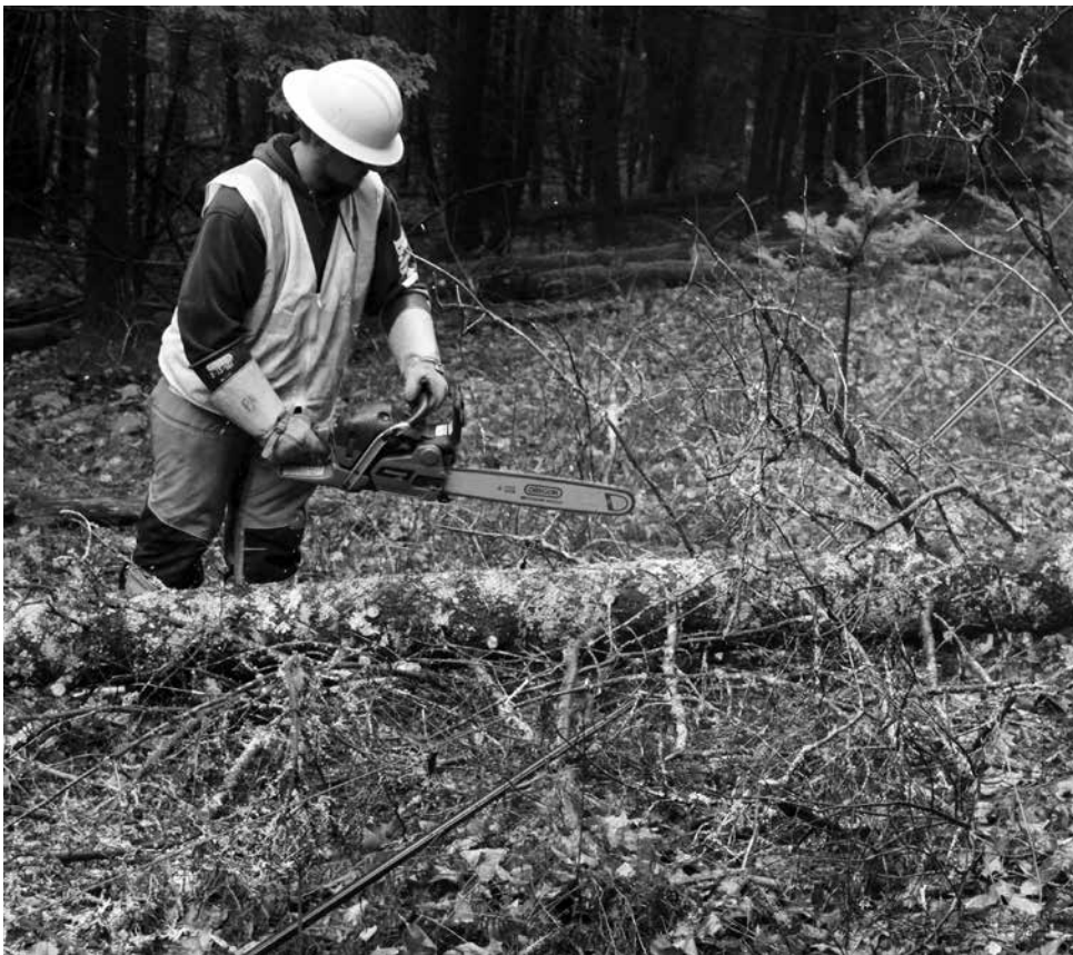
Patrick Morrissey, Apprentice Lineworker. For members without power, the roar of chainsaws was a hopeful sound.
