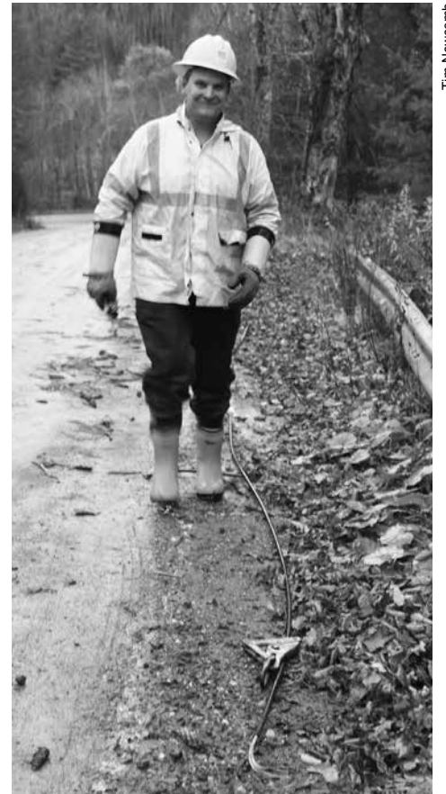
Apprentice Lineworker Nick LeBlanc inspects a downed line on Hampshire Hill Road in Worcester.
