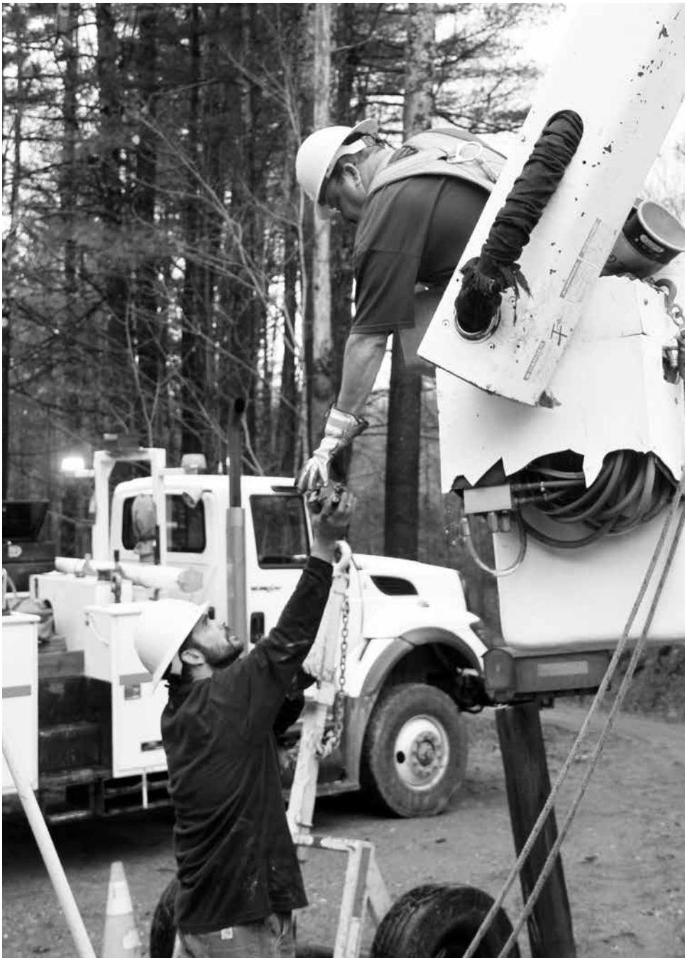
Donnie Singleton (L) and Larry Gilbert (in bucket) setting a broken pole in Middlesex.
