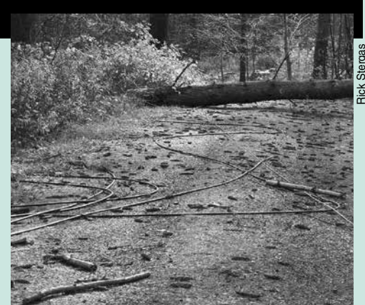
While patrolling the lines, WEC employee Rick Stergas captured this mess of wires on a roadway, pinned under a tree toppled by high winds during the October 30 storm. Read more about WEC’s power restoration efforts on p. 4.
