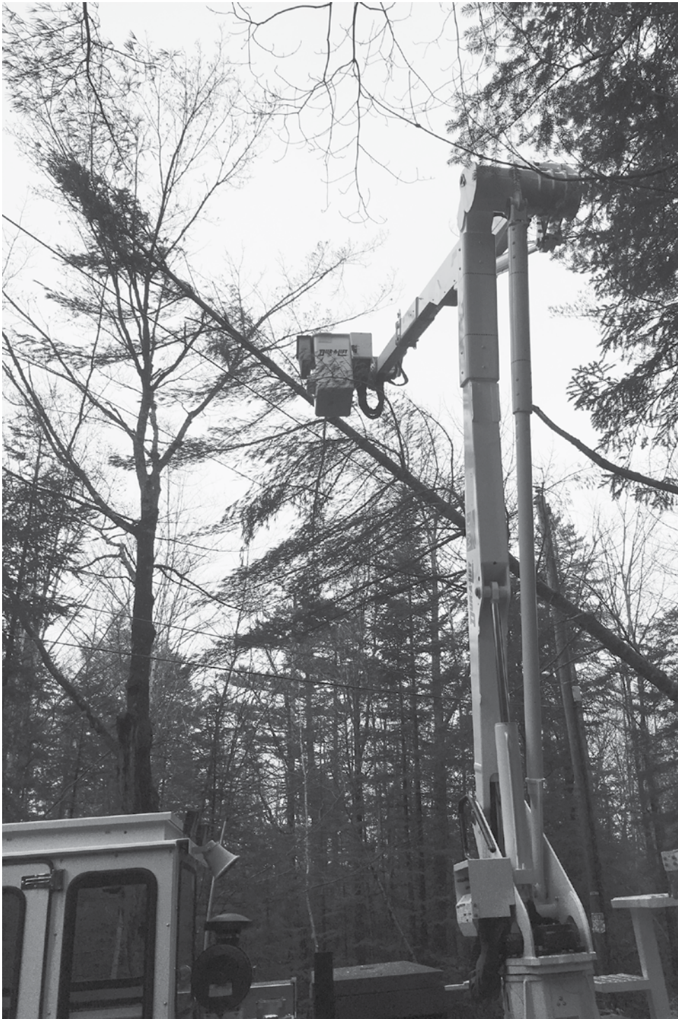
WEC crews go high to take down this very tall, very dangerous tree over the lines.
