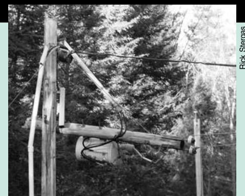
FEMA is reimbursing WEC for 75 percent of the restoration and repair costs associated with the October 2017 windstorm that caused week-long outages and 22 broken poles — like this one. WEC is also receiving funds for future hazard mitigation. Story on p. 2.
