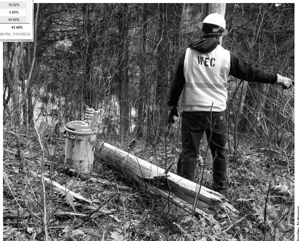
In Stannard, a splintered pole lies on the ground while crews set a new pole. 23 poles broke in the Halloween storm, which may be a WEC record. Broken pole repair takes far longer than line repair because crews need to drill, sometimes through ledge, and set the new pole before they can restrung the wires.
