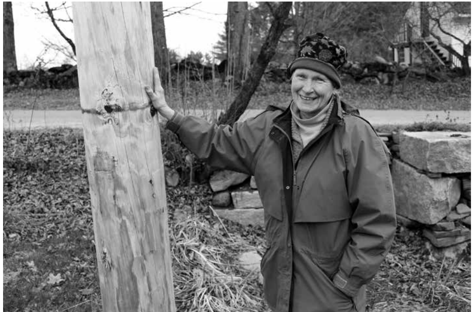
Annie Reed, WEC’s Board Secretary, with the pole that holds her transformer. Some years ago, line crews needed to reset the pole and were careful to set it in a new location that gave her enough room to drive a lawnmower between the pole and the bedrock that lines her garden. “I came out and said ‘Oh, you really get me! This is perfect!’” she said. “They are so kind, so great.”
