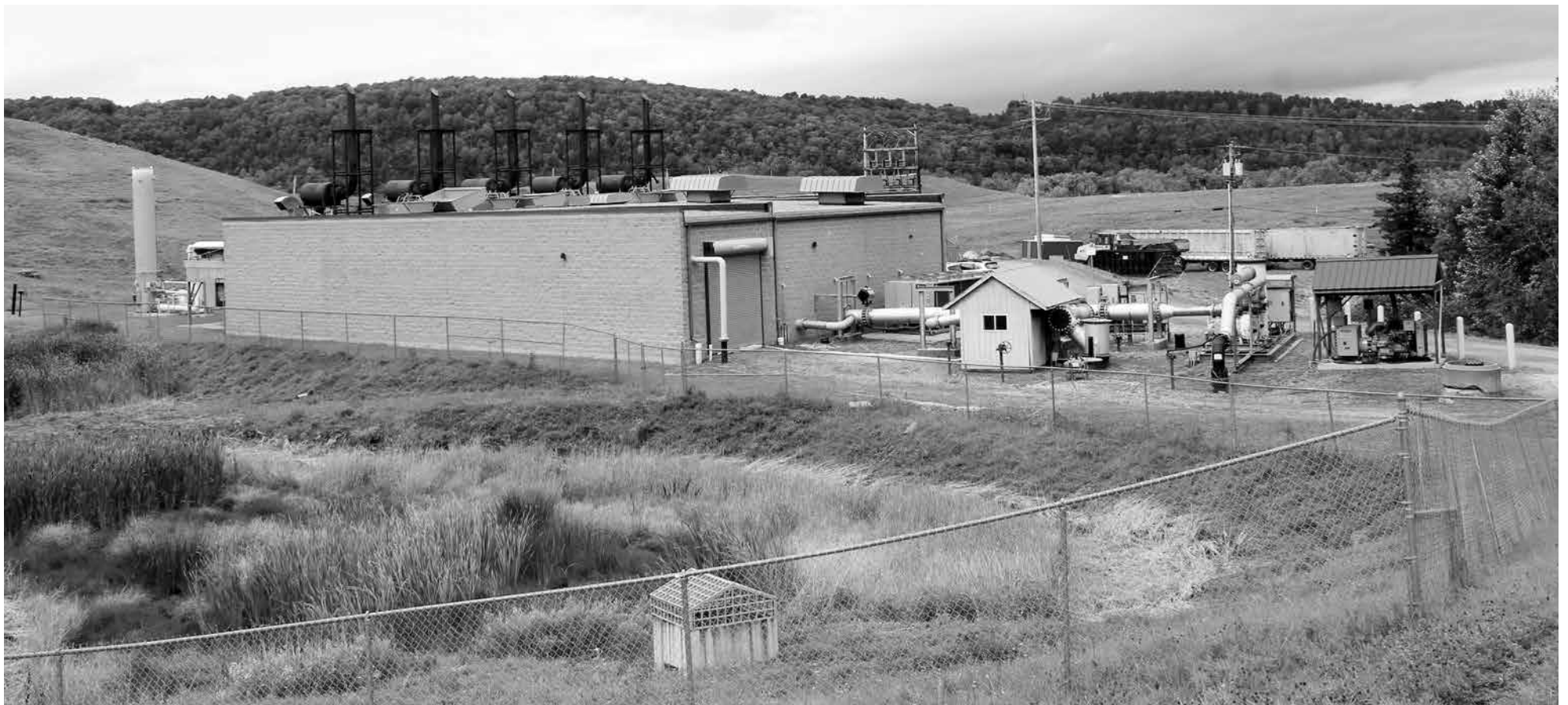
WEC's landfill-gas-to-energy power plant at the landfill in Coventry.
