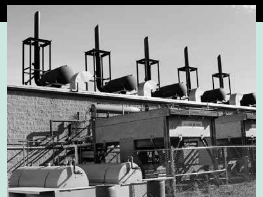
It was a banner year for electricity production at WEC's landfill gas plant at Coventry Landfill. The plant produced enough energy to power well over two thirds of WEC member homes. More in the President's and General Manager's report, p. 2.
