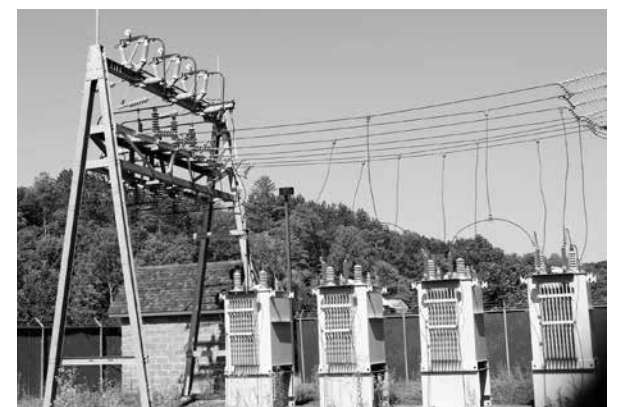
Transmission lines, managed in Vermont by VELCO and GMP, connect into distribution utilities' substations. Here, the voltage is stepped down and sent out on three-phase and single-phase lines. Each substation powers many miles of distribution lines, so if a transmission line goes out, the substations connected to it lose power—and so do thousands of members.
