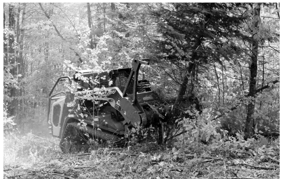
In 2021, WEC's forestry head skid steer cleared just over 26 miles of dense brush in the Co-op's Rights-of-Way. That's approximately the same distance as a marathon.
