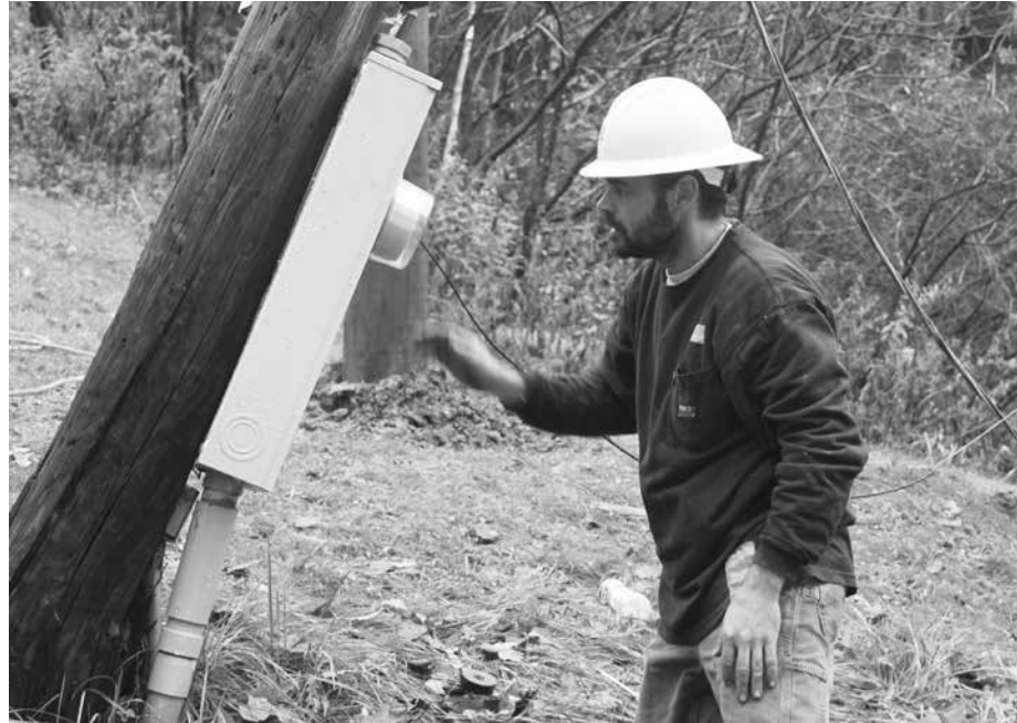
Lineworker and Equipment Operator Donnie Singleton works to set a new pole. Increased funding access for Communications Union Districts (CUDs) changes the nature of the partnership between CUDs and WEC, allowing broadband deployment to continue without the Co-op taking on additional debt. WEC will concentrate on doing the necessary work to prepare its poles and Rights-of-Way for installation of fiber by the CUDs.
