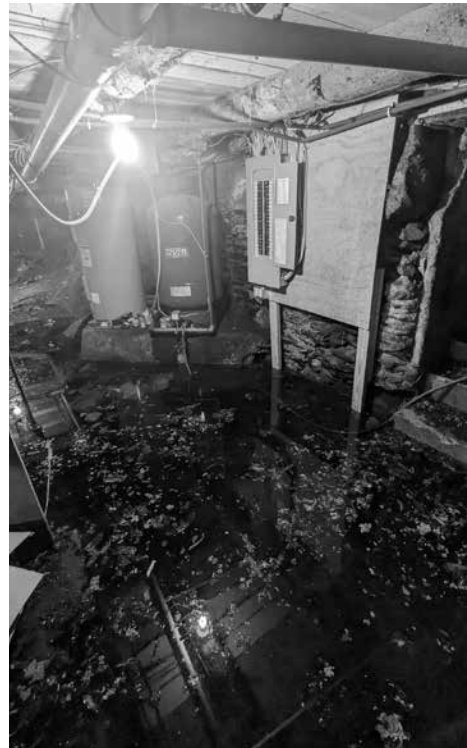
Many Vermonters experienced flooded basements this July, including Operations Assistant Kayla Dunbar.
